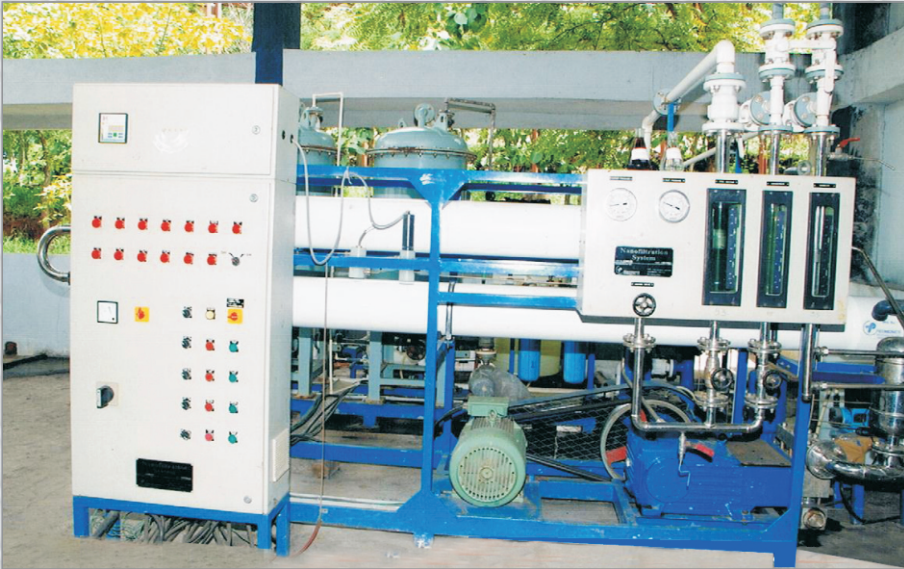
Nano Filtration system Effluent Treatment Plant
